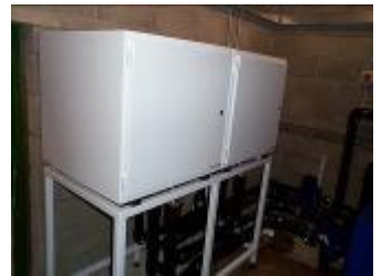
Communal Heat Pump System
