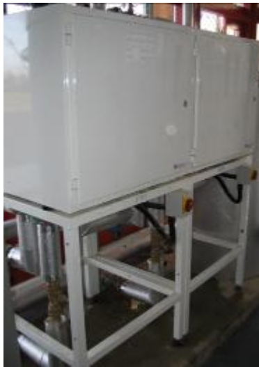
Fig 6 Plant room heat pumps
