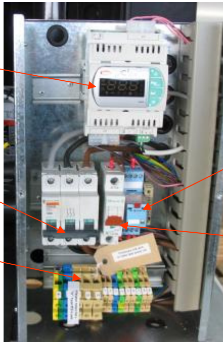
Fig 9 Electrics box with the front removed
