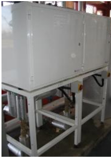
Fig 6 Plant room heat pumps
