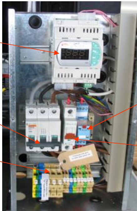
Fig 9 Electrics box with the front removed
